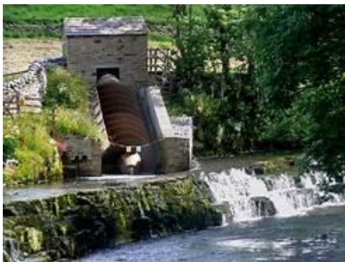
Archimedes Screw electricity generator
